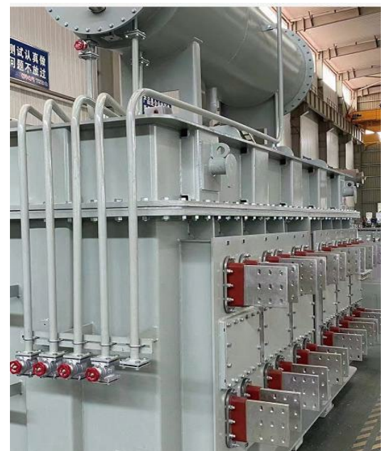
>110kV furnace transformer
